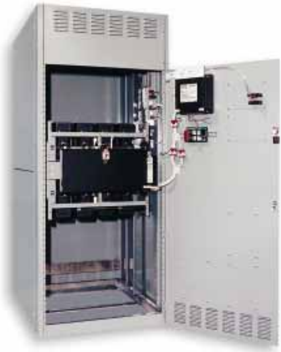
Fig. 3 Delayed Transition Transfer Switch rated 4 pole 1200 amperes.
